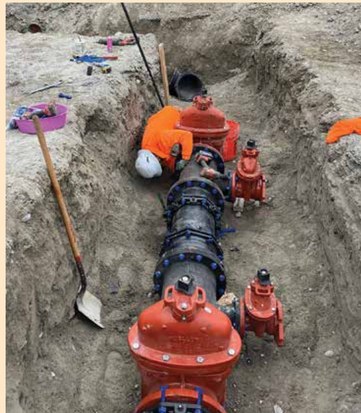
As with all of our projects, if water service to a residence or business will be impacted for any duration during construction, we will notify them several days in advance with an estimated time they'll be without water. Should you have any questions about these projects, feel free to give us a call at 206.362.8100.
